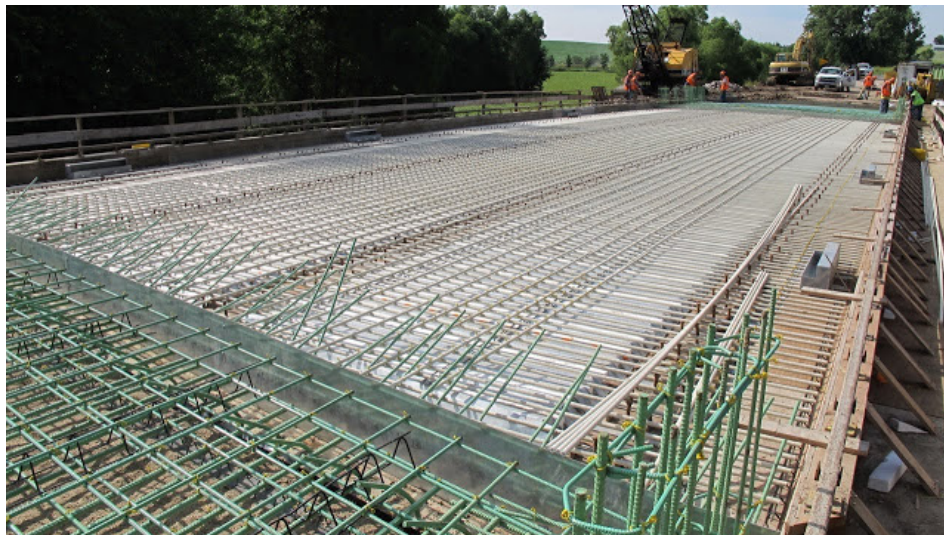
Bridge construction in the US using GFRP rebars. Photo courtesy of Hughes Bros.
