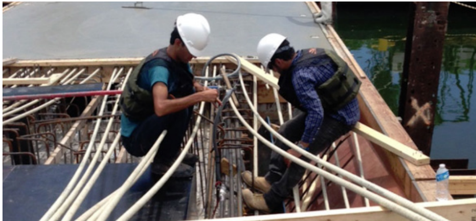
Students at University of Miami replace steel with GFRP on bridge research project. Photo: Composites Manufacturing; University of Miami
